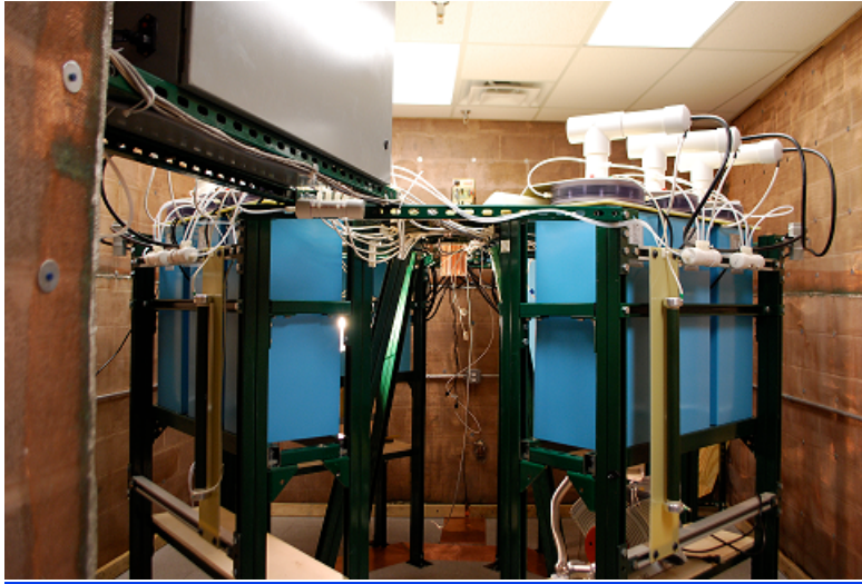
The Focus-Fusion-1 Dense Plasma Focus, shown here before installation of the vacuum chamber, concentrates energy stored in an 8- foot wide array of capacitors (blue) into small copper electrodes (center).
